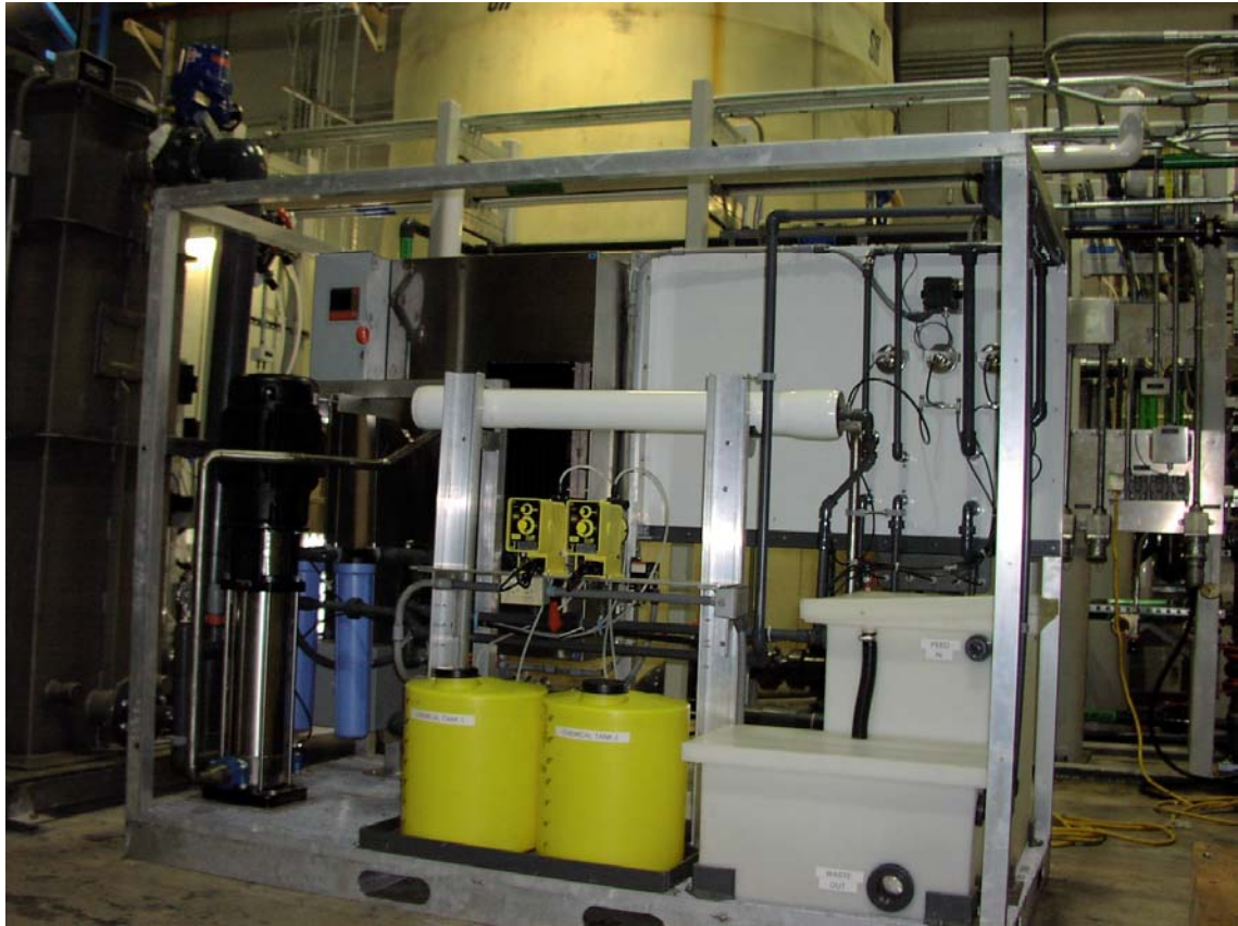
Figure 2. Black & Veatch RO Membrane Pilot Unit.
