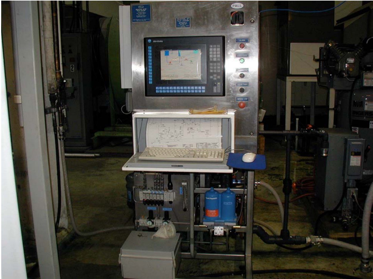
Figure 2. MF Unit PLC and Operator Interface
