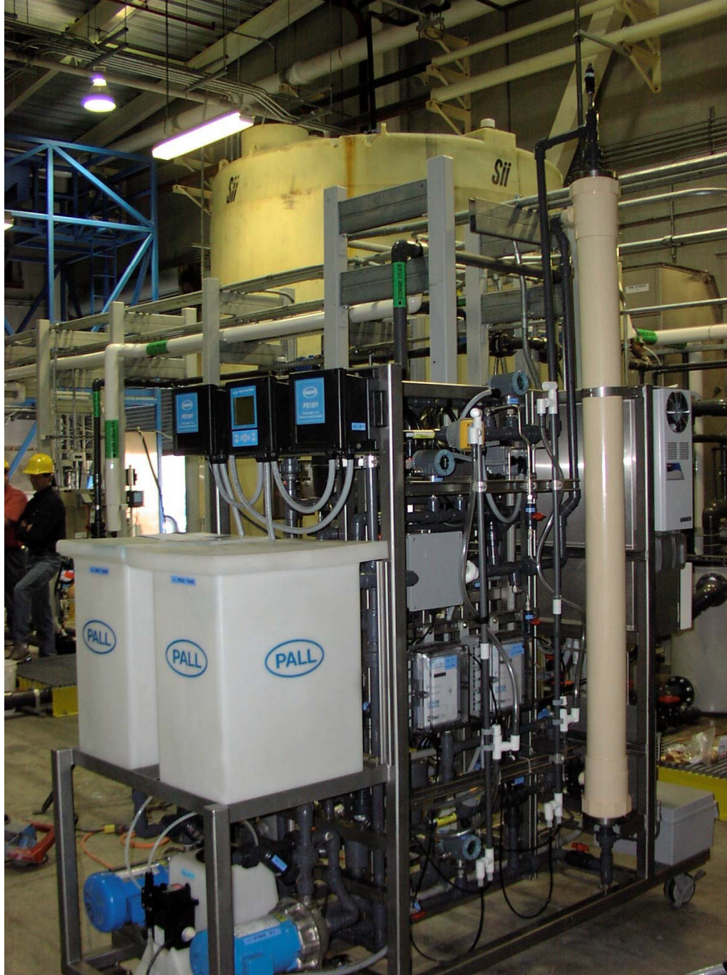
Figure 2. Pall Microfiltration Membrane Pilot Unit.
