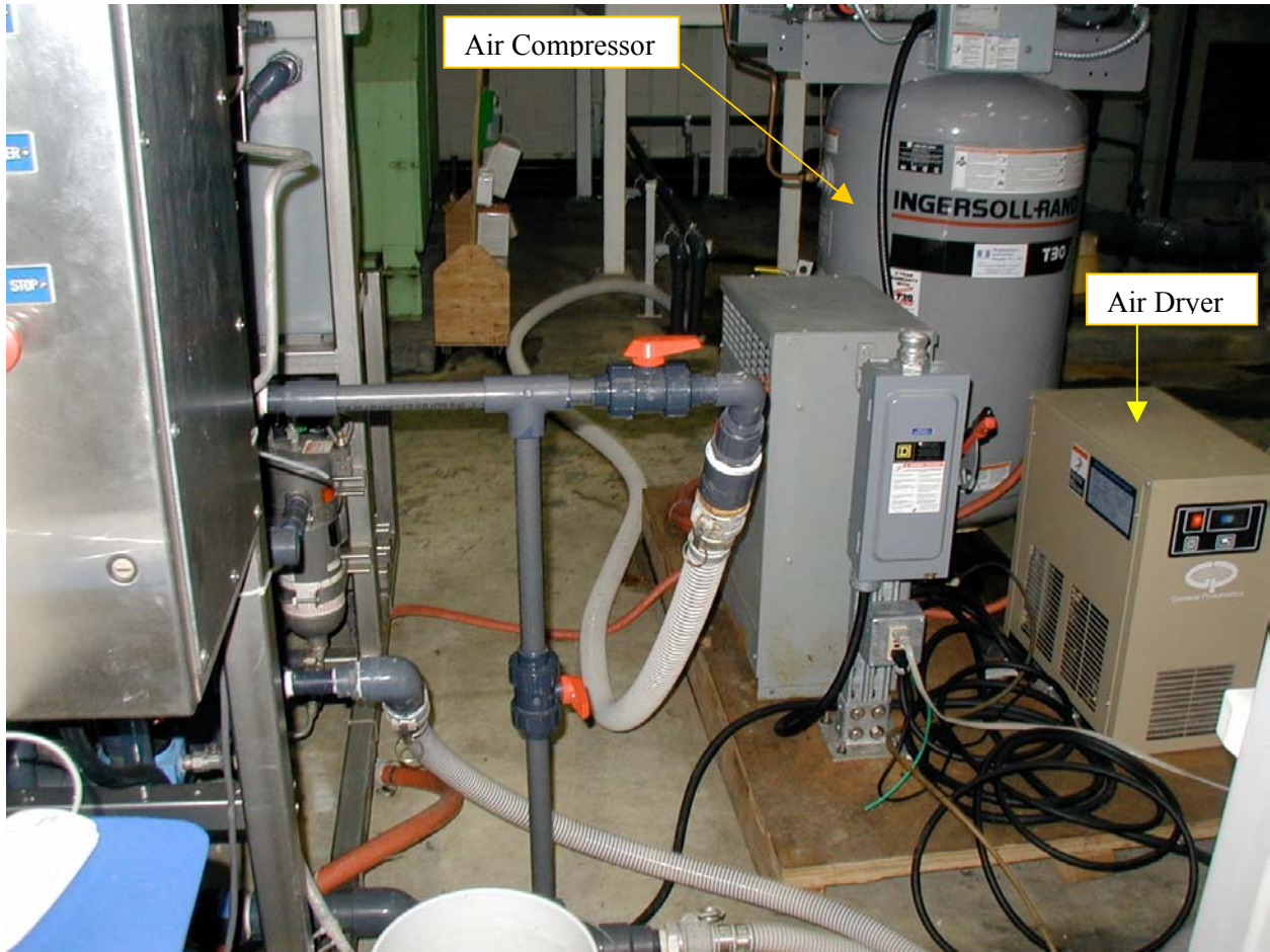
Figure 4. MF Pilot Unit Air Compressor Skid
