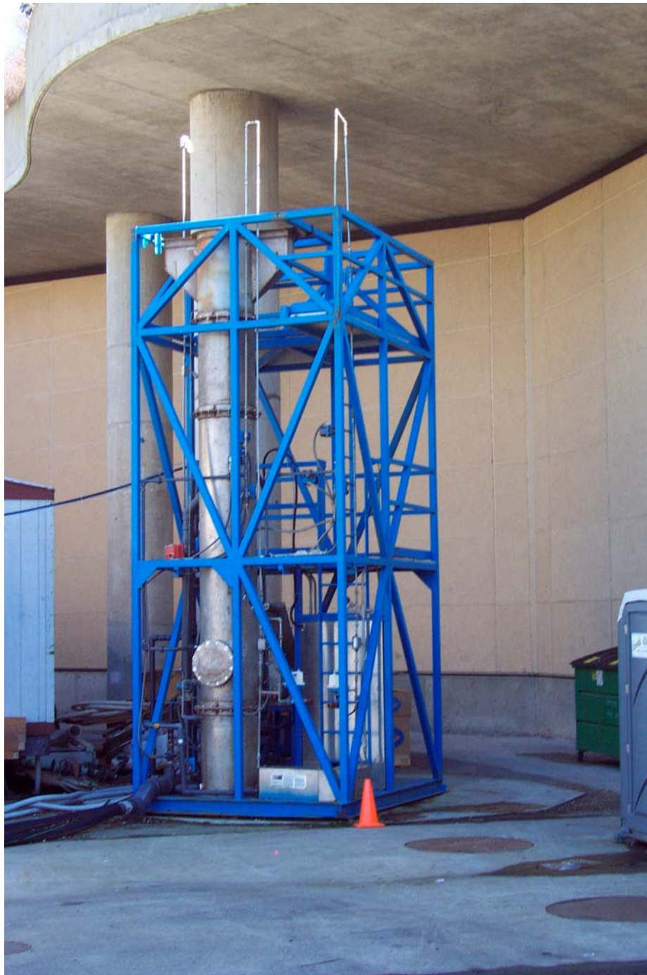
Figure 3. BAF #2 Pilot Plant at Westpoint Wastewater Treatment Plant
