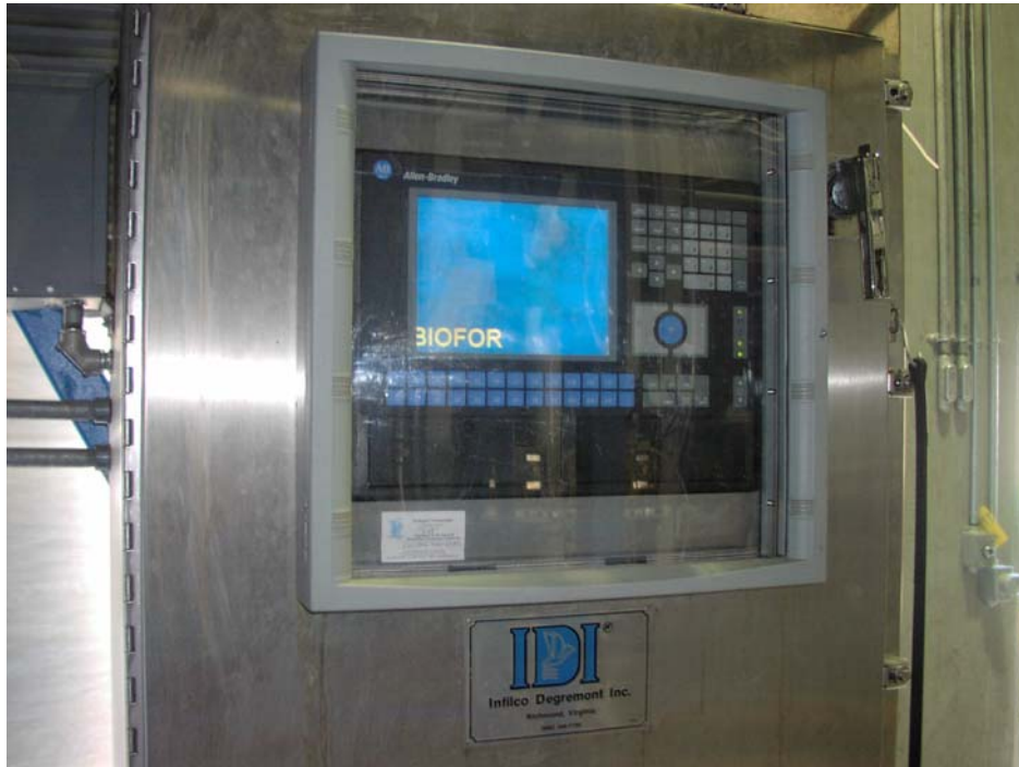
Figure 6. BAF #1 Panel PC (Control Interface)
