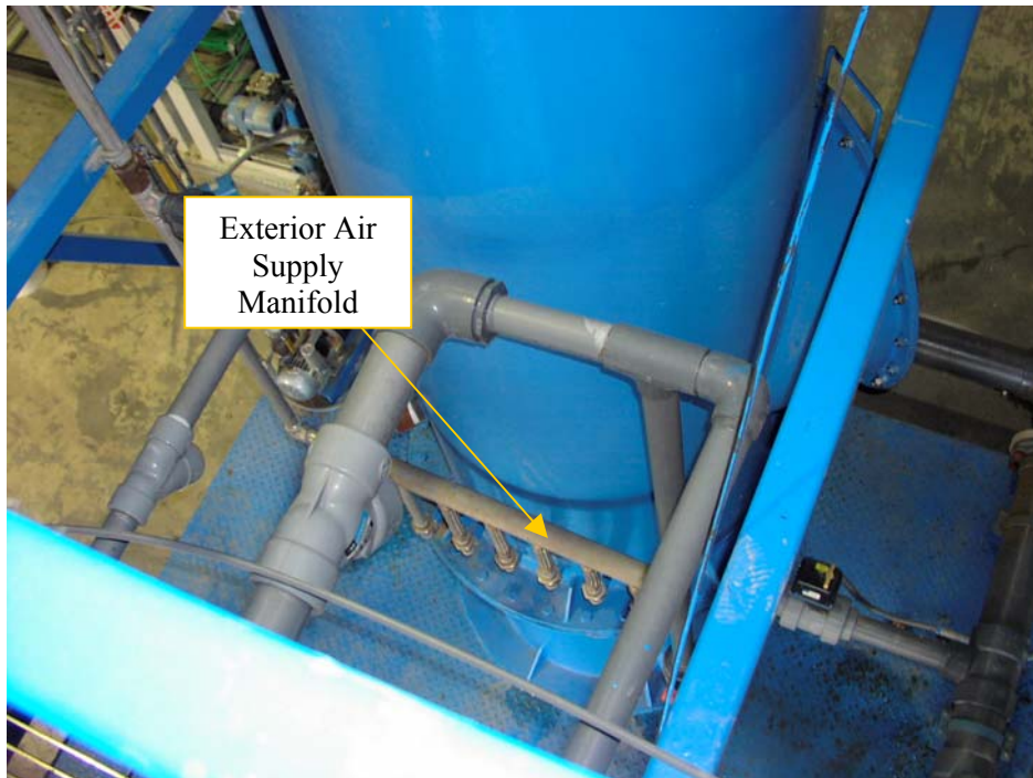
Figure 3. Exterior Air Supply Manifold
