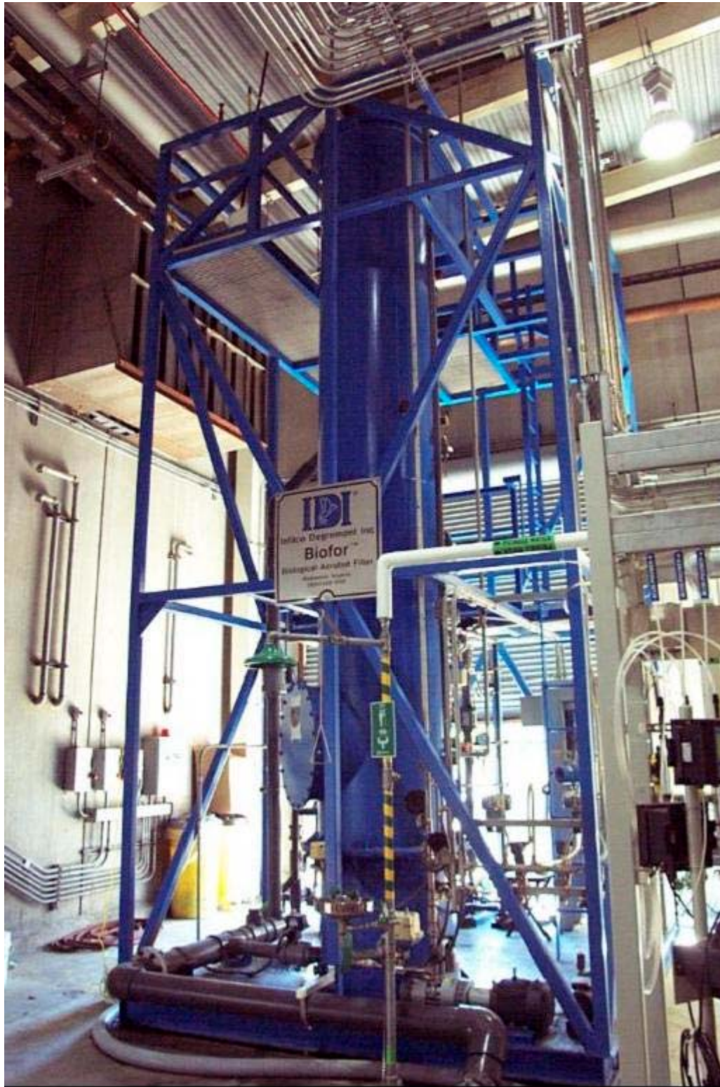
Figure 3. BAF #1 Pilot Plant at Westpoint Wastewater Treatment Plant
