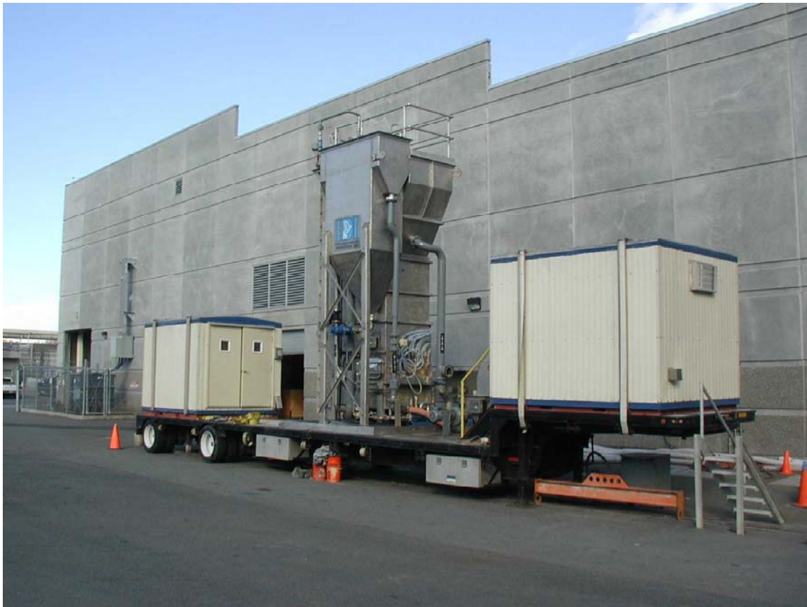
Figure 2. Trailer Mounted Densadeg® Pilot Unit.
