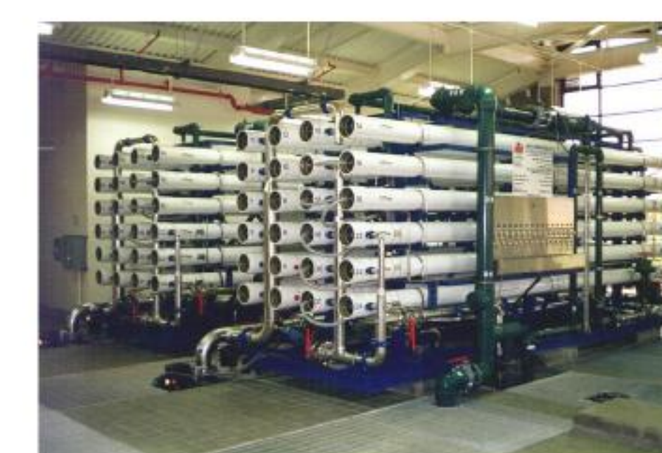
Nanofiltration - Reverse Osmosis
