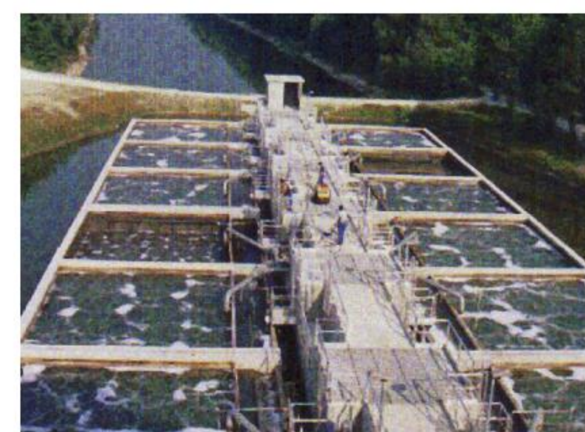
Biological Aerated Filter
