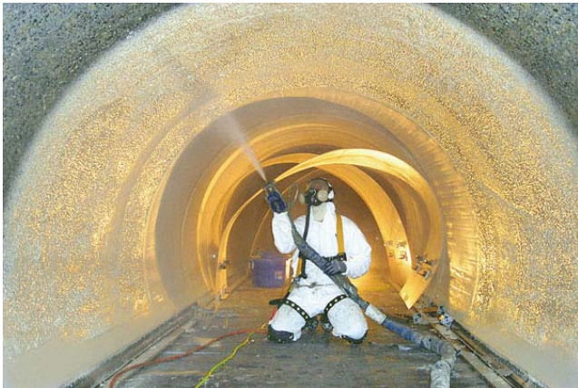
Figure 1-7. A construction worker applies part of plastic liner inside a corroded sewer pipe.
