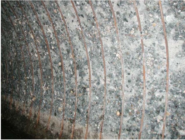
Figure 1-6. Years of exposure to wastewater and hydrogen sulfide gas (H 2 S) have exposed reinforcement bars in some sewer pipes.
