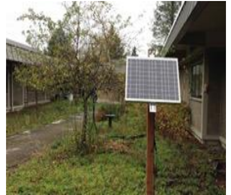
Solar panel powers the cistern water pump in the school garden
