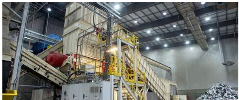
Figure 5-1: Waste processing equipment at the Edmonton Integrated Process and Transfer Facility.
