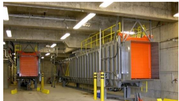
Figure 3-3: SSI 4500 Waste Compactors
