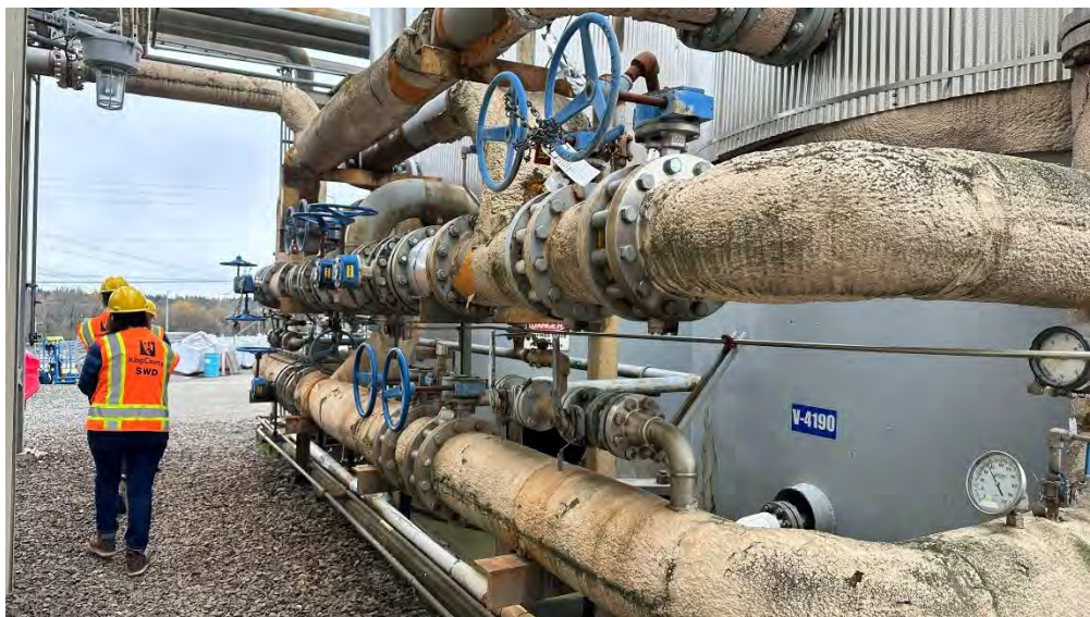
SWD staff walking through the landfill gas plant
