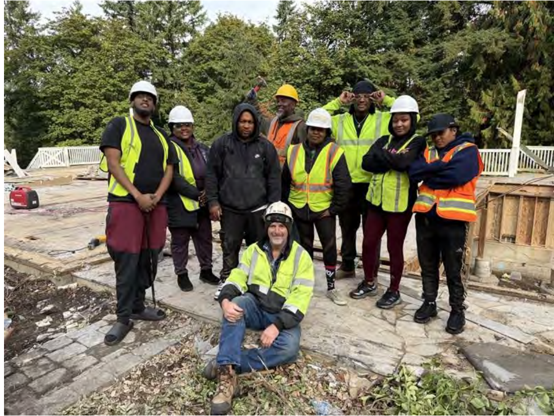
The Solid Waste Division is building a workforce trained in deconstruction, an effective alternative to demolition that dramatically reduces the amount of worksite material that ends up in the regional landfill.
