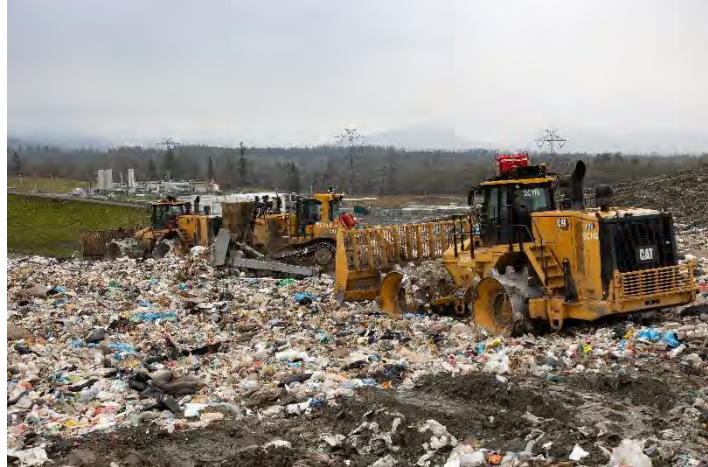
Trash being compacted at the active area of the Cedar Hills Landfill.
