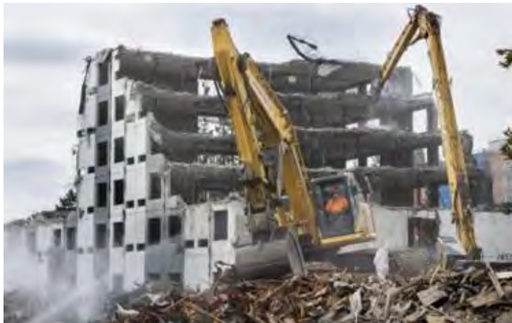
This Bellevue hotel is an example of conventional demolition that using heavy equipment.
