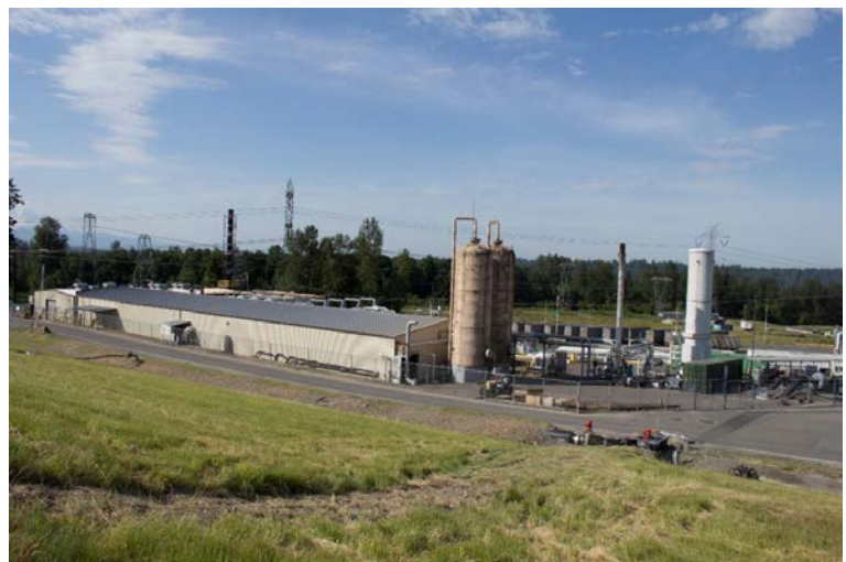
The onsite Bio Energy Washington facility processes landfill gas into a renewable energy source.
