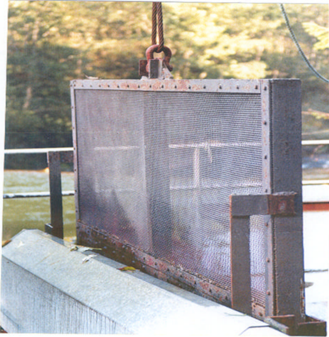
Figure Pass-8. Backup intake screen, Tacoma Headworks diversion dam. (Source: Tacoma Public Utilities)
