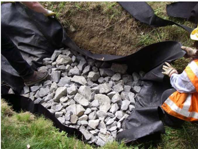
Figure 4. Splash pad trench lined with geotextile fabric, filled with angular rock mixture, and wrapped inward over the splash pad edges, which is then secured with angular rock.
