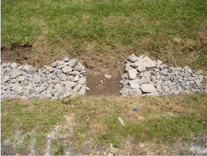
Figure 5. Lower rock ramp and upper rock ramp installation with 2-foot long gap left to allow for treatment cell installation.
