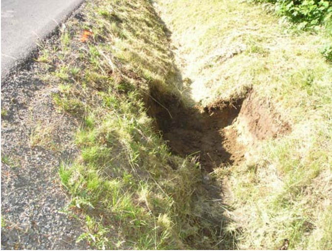
Figure 3. Ditch section prepped for BMP placement with excavations for spill pads. Lower end of ditch looking east.
