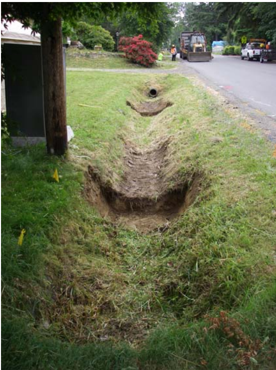
Figure 3. Ditch section prepped for BMP placement with excavations for spill pads. Lower end of ditch looking east.
