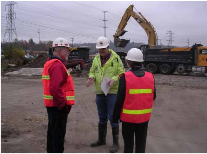
North Wind's Wier off-channel habitat construction in Tukwila is one of the first projects of the Green/Duwamish Ecosystem Restoration. Cleanup of contaminated soils began in 2004. November 2004 photo.
